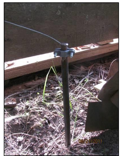
Grounding rod photo courtesy of Gillian Sanders
